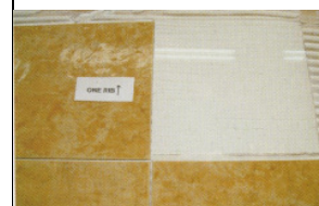
Movement in substrate affects installation of ceramic tiles.
